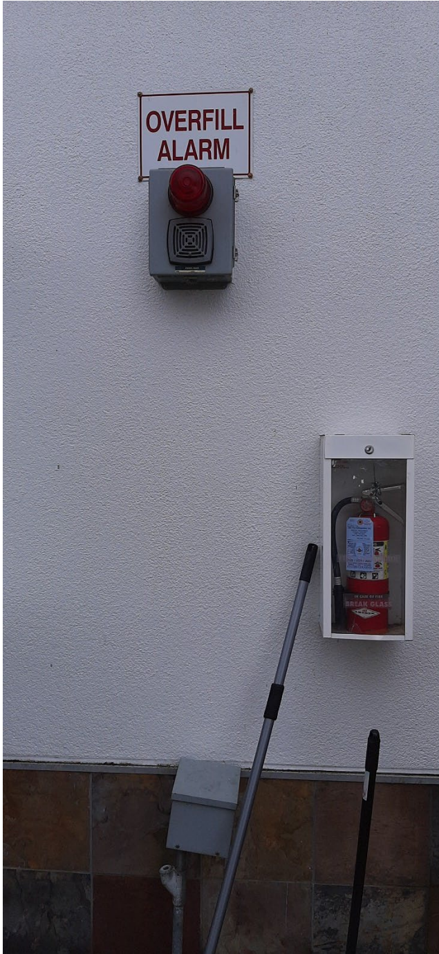
15: Overfill alarm east side of building
