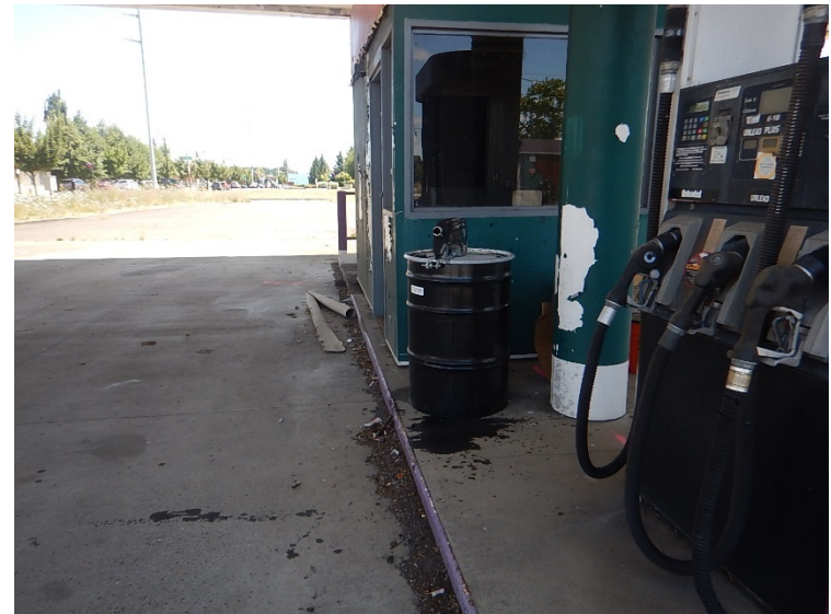
View of general area of soil gas sample SG05, placed beneath the fuel island canopy.
