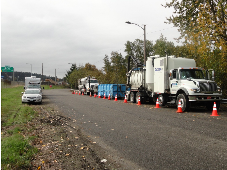
P-9: Vac-truck, jet-truck, and sediment roll-off box staged on Glass Plant Rd east of Johnson Lake.
