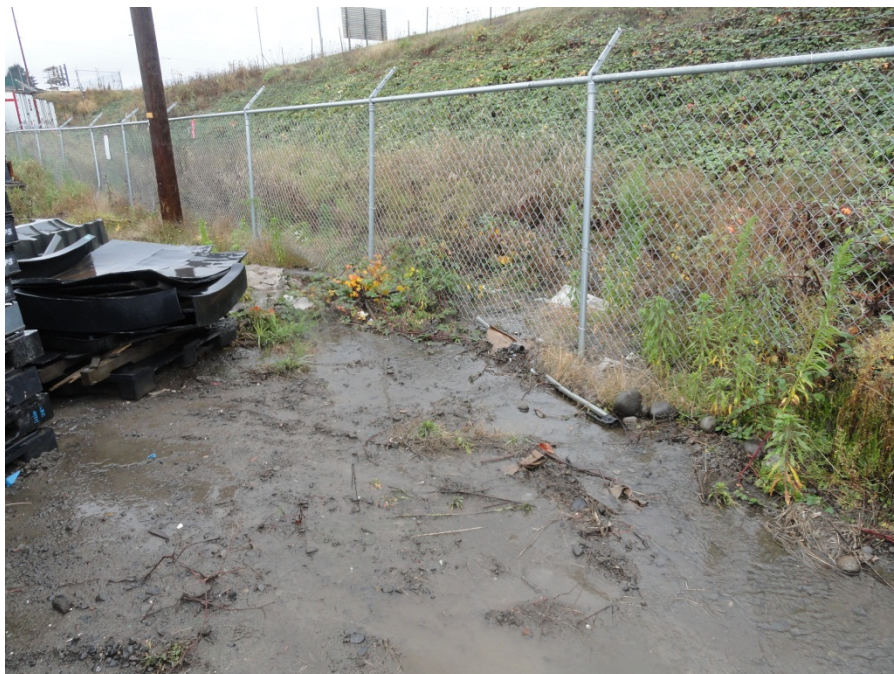
P-8: Storm water runoff on Myers Container property to culvert inlet observed during a rain event.
