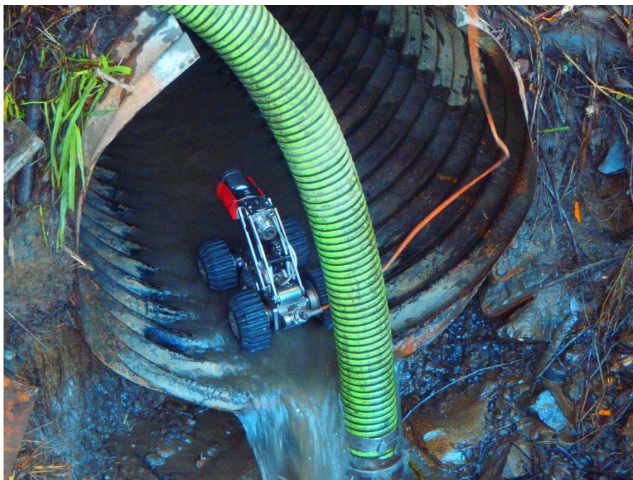
P-10: Remote controlled wheel camera unit enters the culvert to perform post cleanup inspection.
