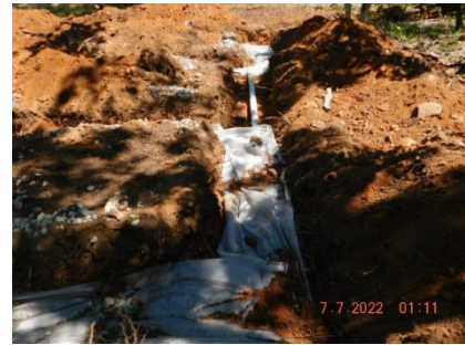
Crossover between Loop 1 and Loop 2
