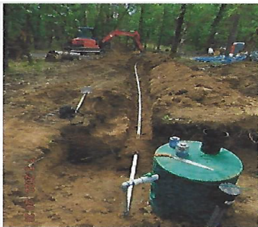
Effluent Line from tank
