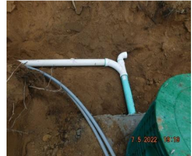
Inlet coming from house
