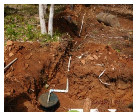
Effluent line into Drop Box
