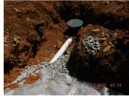
Drop Box 4" pipe to drainfield
