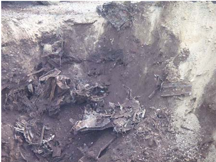
Photograph 9. June 22, 2014 – Initial excavation west end of Phase 1 excavation area; exposed metal waste debris.
