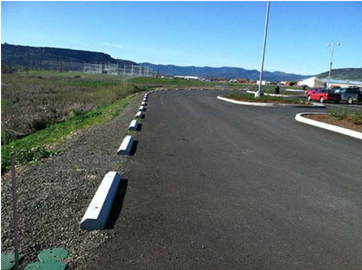
Photograph 35. March 18, 2015 – Completed expansion area parking lot; looking north along west side of new parking lot.
