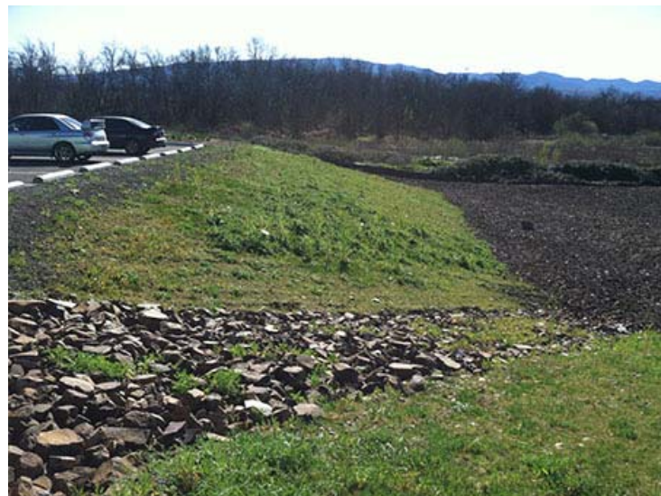
Photograph 38. March 18, 2015 – Completed expansion area parking lot; looking west at area just north of new parking lot.
