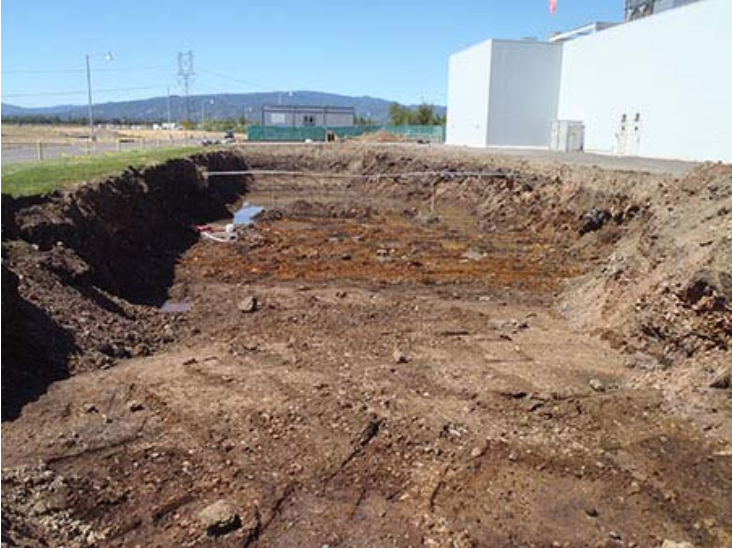
Photograph 12. June 23, 2014 – Initial excavation of Phase 1 excavation area; looking west. Conduit lines located in central area of excavation.
