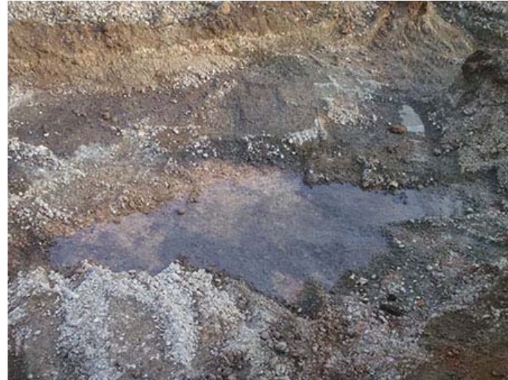
Photograph 22. June 31, 2014 – Final excavation of Phase 1 excavation area; seep water on excavation floor.
