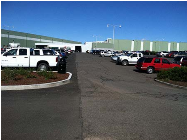
Photograph 34. March 18, 2015 – Completed expansion area parking lot; looking east at old and new parking lot asphalt line.
