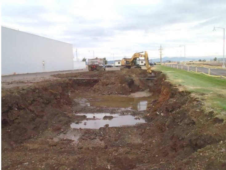
Photograph 11. June 22, 2014 – Initial excavation west end of Phase 1 excavation area; looking east. Conduit units partially exposed.
