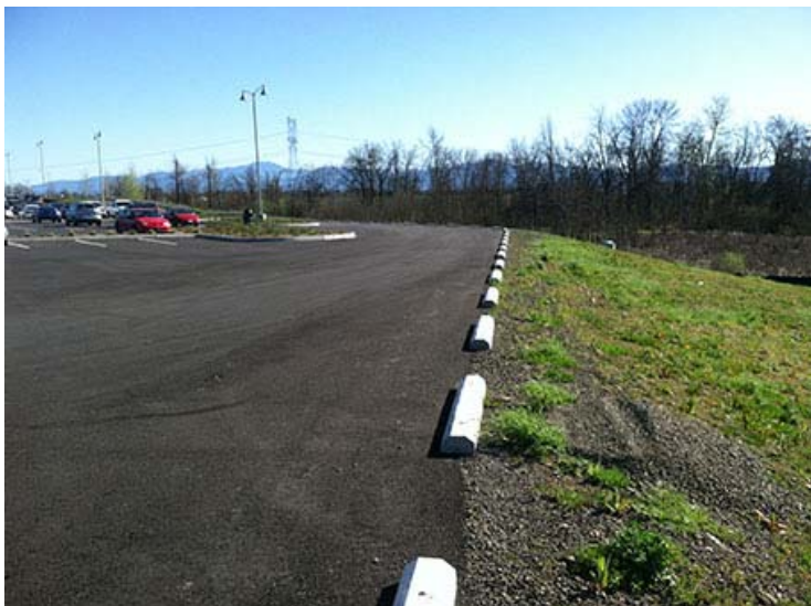
Photograph 37. March 18, 2015 – Completed expansion area parking lot; looking west along north side of new parking lot.
