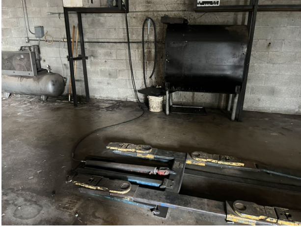
7. The Subject Property – former garage shop interior, above ground hoist and AST, presumably waste oil.
