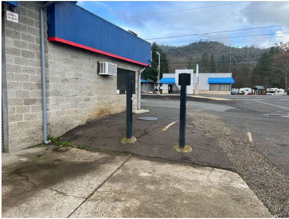
1. The Subject Property and Neighboring Properties - view to the east, note the backfilled pipe trench.
