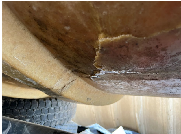
17. The Subject Property – Close up of puncture in the number 3 gasoline UST, likely associated with installation of a new pump that was immediately followed by a water alarm.
