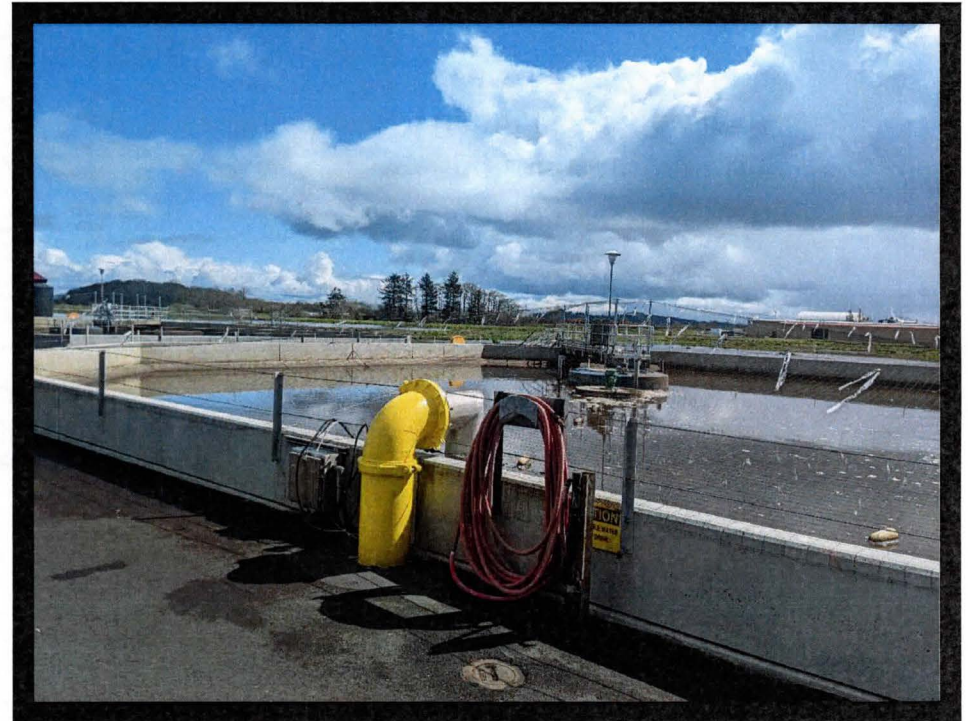
One of 3 SBR basins at the plant.
