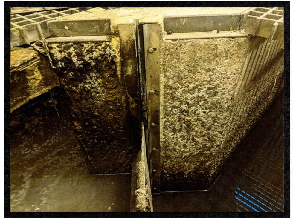
Deteriorated concrete at the headworks channel
