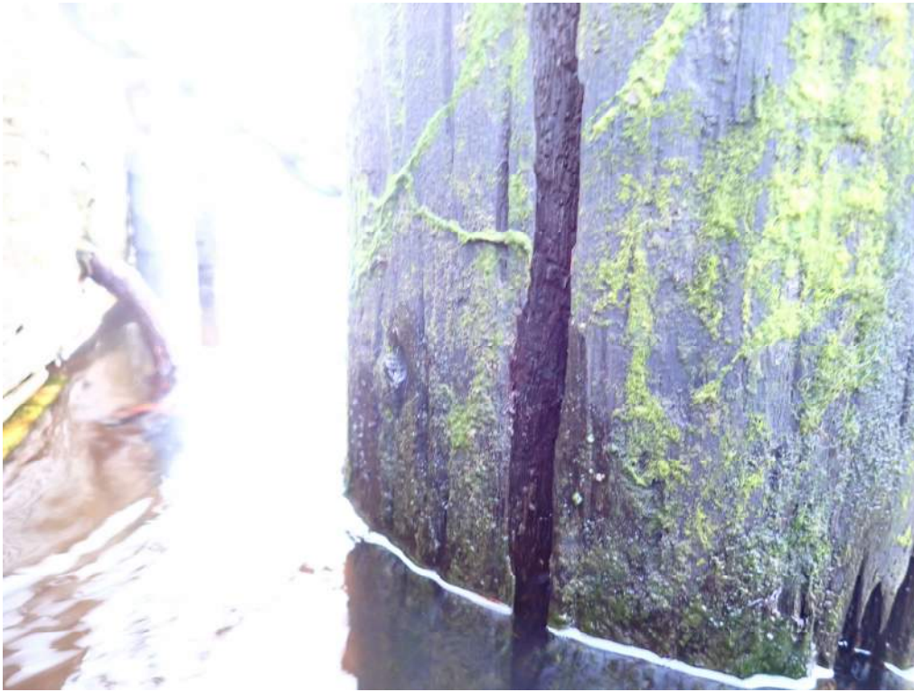
Photograph 27– Typical Check in Timber Piles
