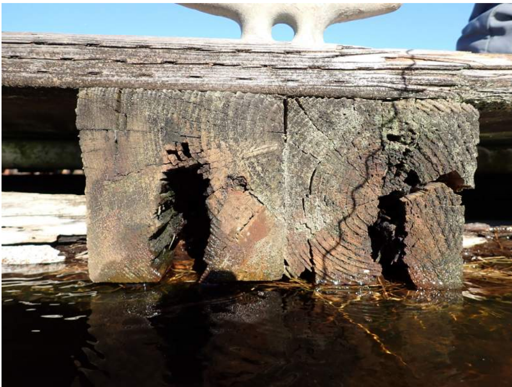
Photograph 28– Typical Section Loss in Timber Transverse Supports
