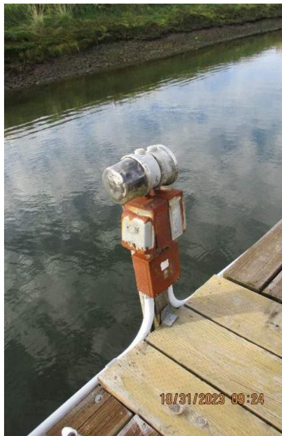
Photo 22: Typical utility pedestal.
