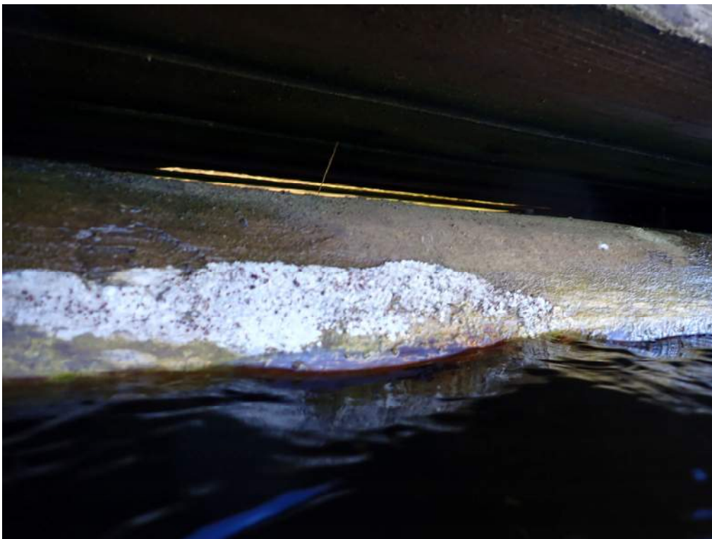
Photograph 14– Typical Timber Float at Waterline
