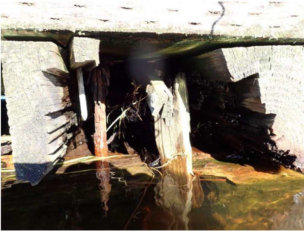
Photograph 29— Loose Connection Between Timber Float and Transverse Timber Support
