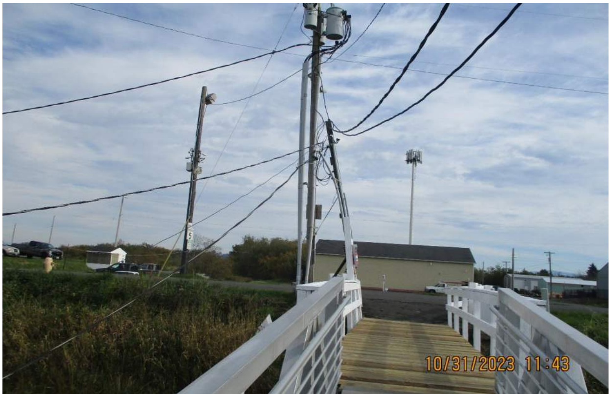
Photo 16: Handrail being pulled down by utility pole.
