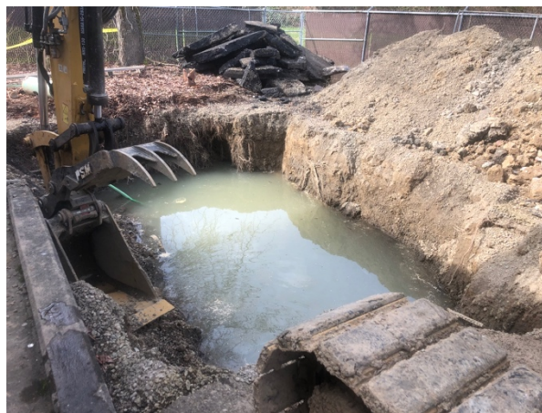
Photo 18. Groundwater in tank pit. Sample WG8@5 was collected from this water. View is to the SW.
