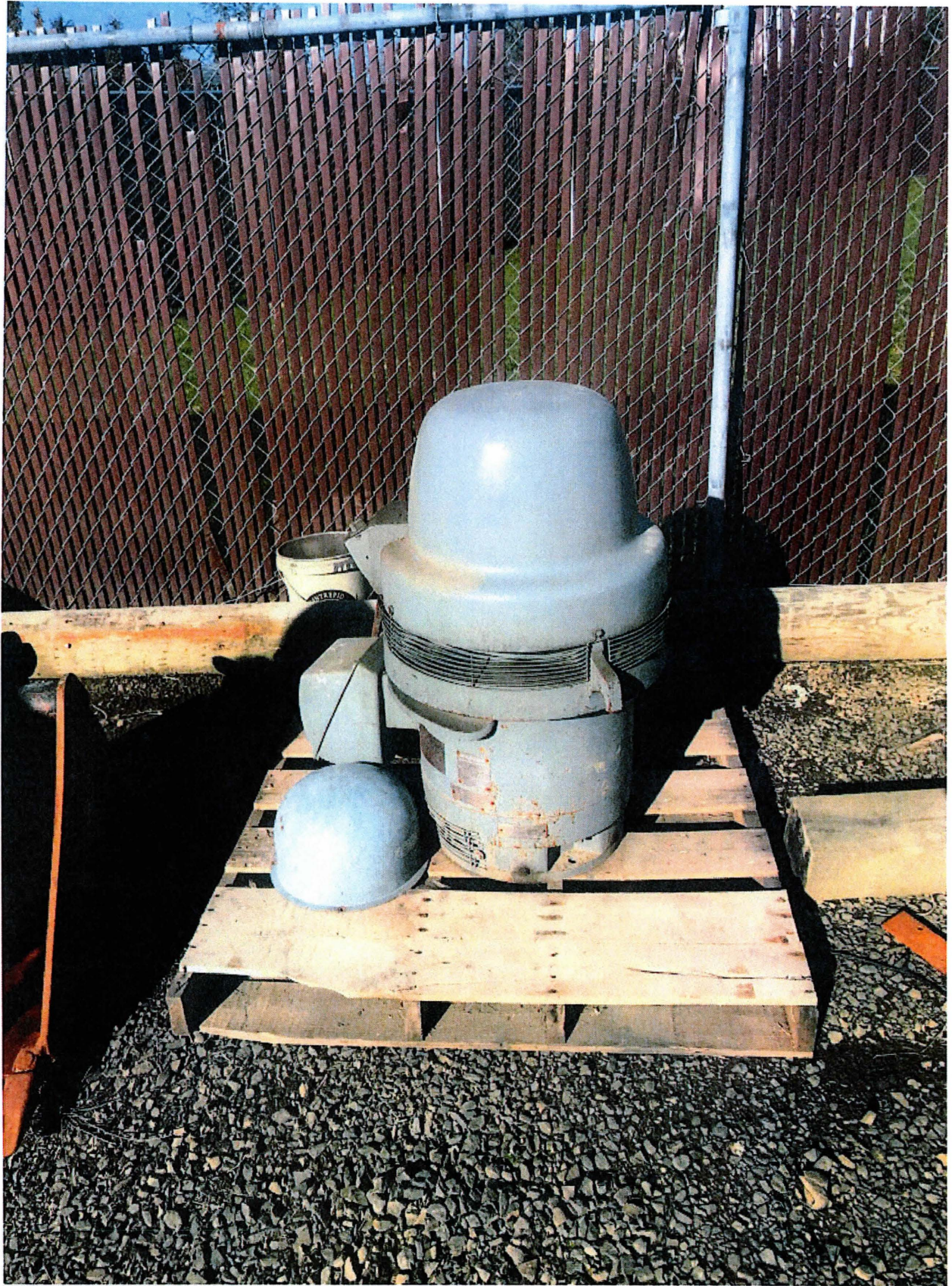
GE Pumpstation Motor
