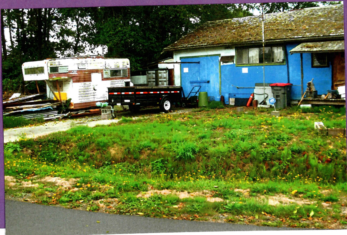
9 th and South Main Avenue, Warrenton this property has been a danger and unsightly for years. The man that “inherited” the property has worked trying to clean it up. But, now the roof has caved in and it simply looks horrible and dangerous.
