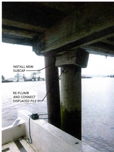
10 PHOTO - WORK PIER DISPLACED PILE AT WP13/A SCALE: NTS
