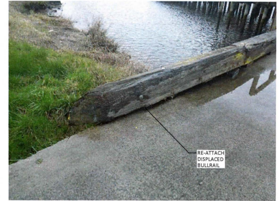
15 PHOTO - DISPLACED BULLRAIL AT ET0.5/B SCALE: NTS
