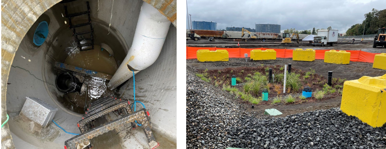
Figure 1. Basin K1 Stormwater SCMs (left: diversion manhole with pump; right: bioinfiltration basin)
