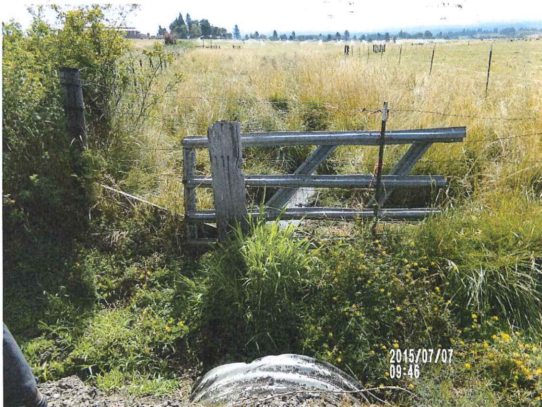
Photo 6. Water flowing from NE corner of Coleman Ranch North property into culvert.
