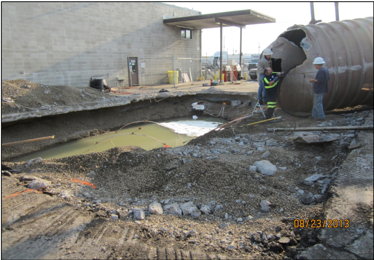
Photograph 3. Tank Pit after removal of first tank, note deployment of absorbent pads, fractured tank. 8-23-2013.
