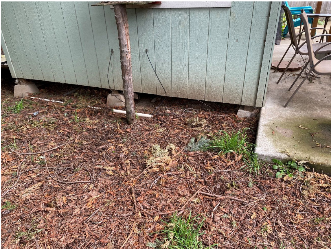
Photograph shows the west side of the ADU in the northeast corner of the backyard. Photograph facing northeast.
