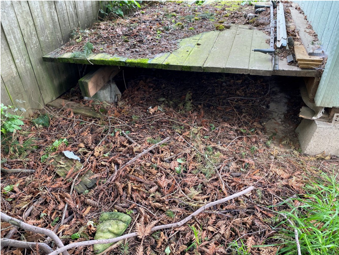
Photograph shows the west side of the deck on the north end of the ADU (to be removed). Photograph taken facing east.
