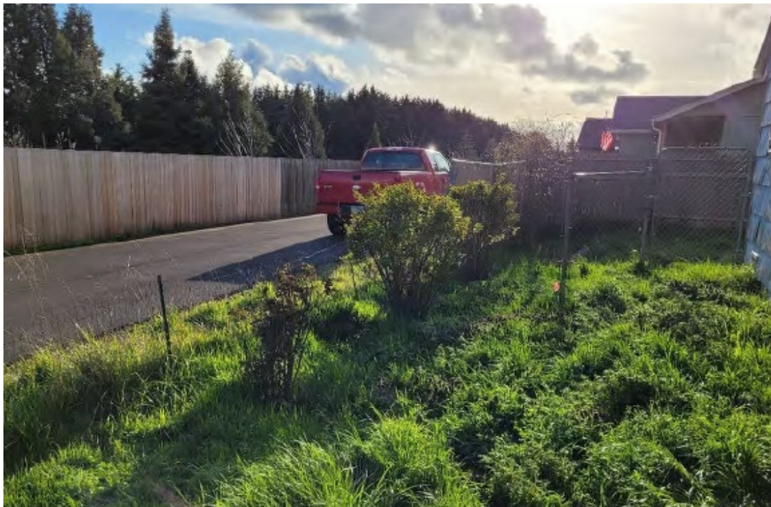
Photograph shows shrubs to be removed prior to remedial action and replaced from the south property line. The fence will need to be removed for equipment access. Photograph taken facing southwest.
