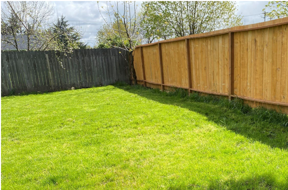
Photograph shows more of the south fence to potentially be removed/replaced. Photograph taken facing southeast.
