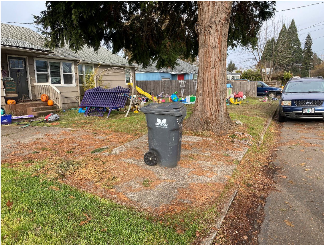
Photograph shows the front yard of the property. The large cedar tree will be left intact. The driveway of this property will be removed to access soil underneath. It will be covered with bare soil following remedial action. Photograph taken facing northwest.
