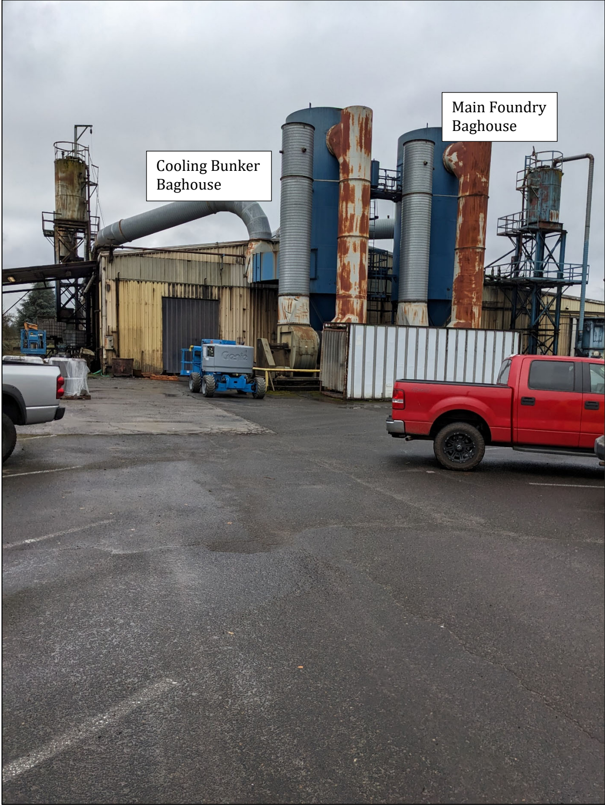
Figure 1 Main Foundry and Cooling Bunker Baghouses
