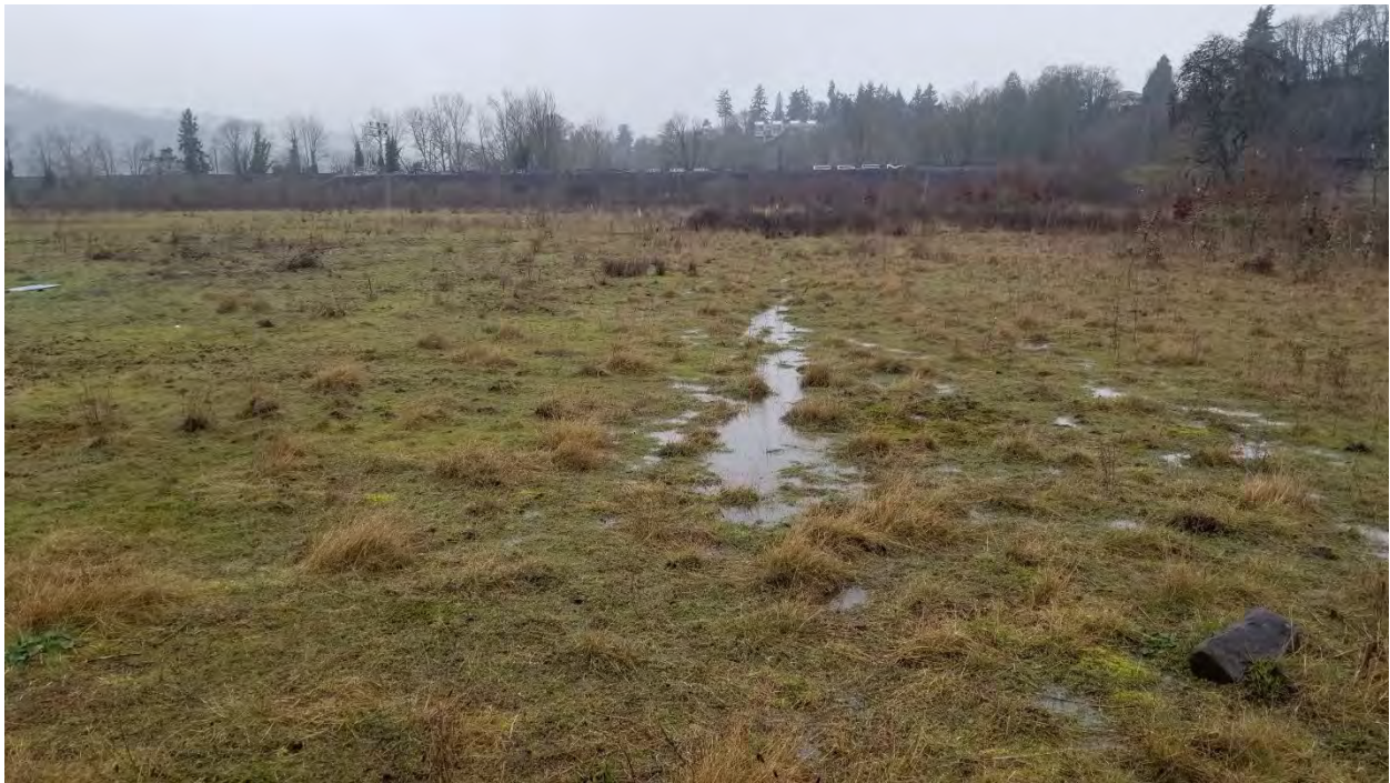
Photograph 8: Standing water on the soil cap just to the east of the surface trace of the barrier wall between MW-51s and MW-53s.
