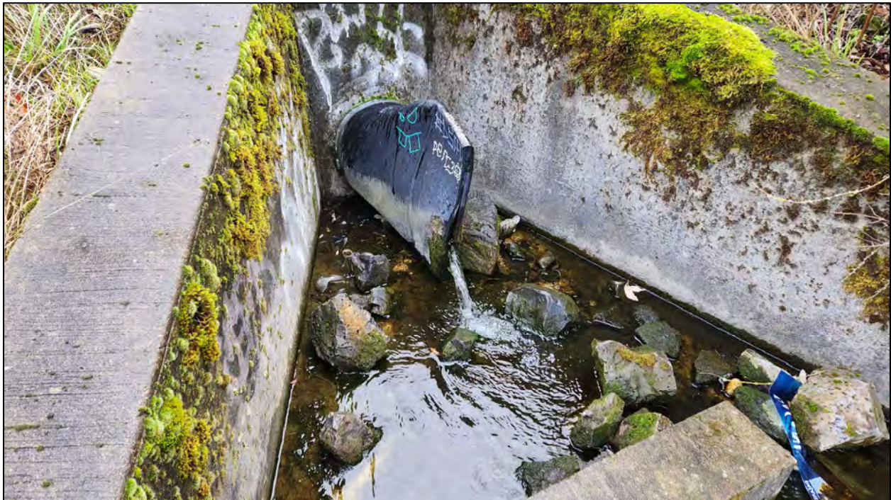
Photograph 4: Water flow (estimated at 20-30 gpm) from the stormwater outfall.
