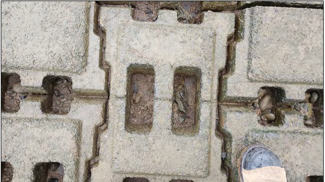
Photograph 2: ACB in Willamette Cove with no sand or river rock occupying the void space.
