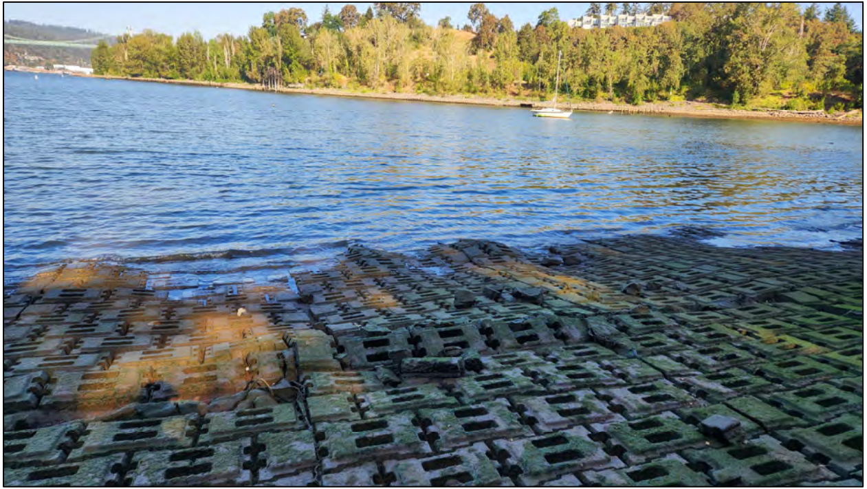
Photograph 3: ACB armoring with unconformities shown along Willamette Cover Shoreline. View facing north.
