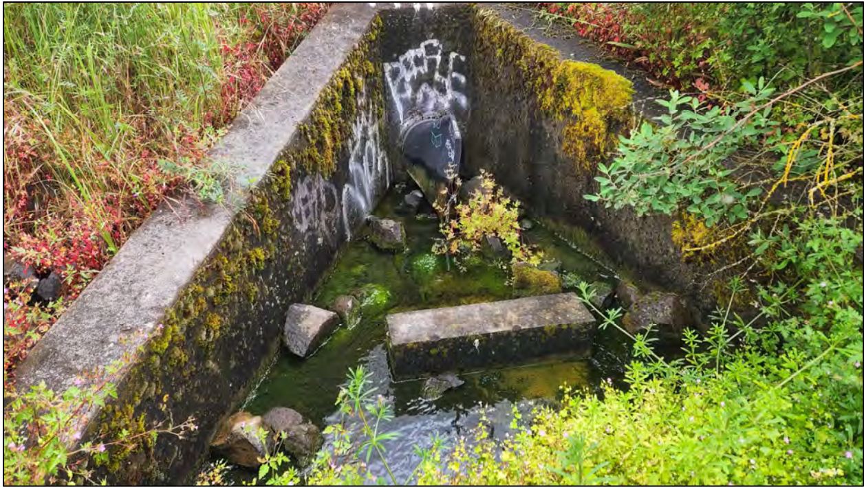
Photograph 3: Stormwater outfall flow at approximately 6 to 9 gallons per minute. View facing northeast.
