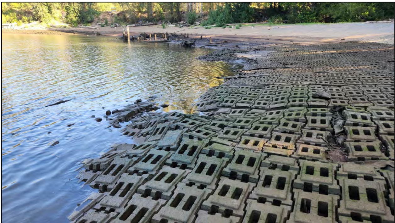
Photograph 2: ACB unconformity with largest amount of observed deflection on eastern end of ACB in Willamette Cove. View facing northeast.
