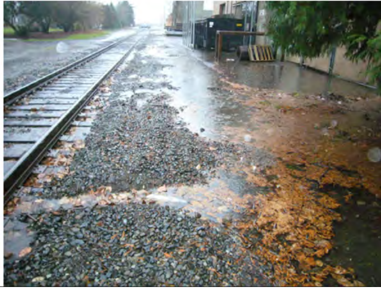
Photograph 1: Extensive Ponding Adjacent to the West Side of the PIW Building and Along the N. Bradford Street ROW circa 2012
