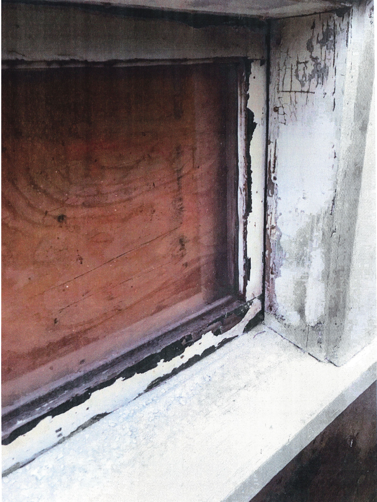
All windows dry rotted with decades of deterioration due to failed caulking.
