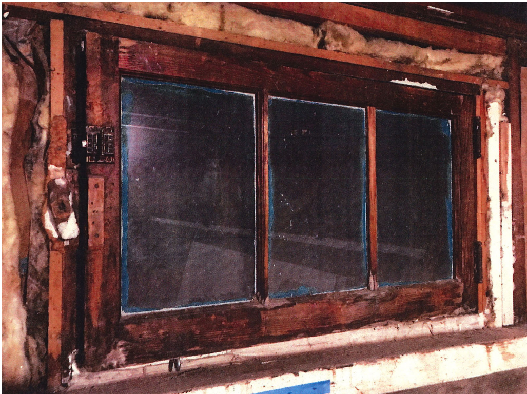
Existing windows all dry rotted, unable to be secured and leaking driven rain into the house.
