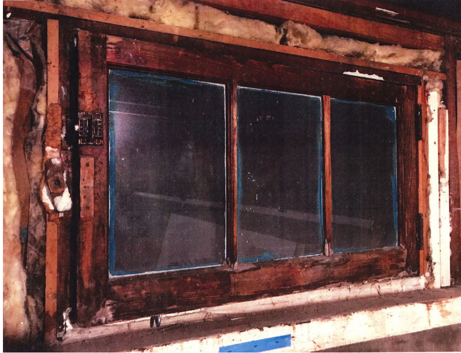
All windows so deteriorated that they are literally rotting off the hinges.
