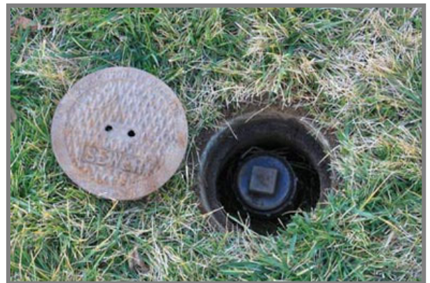
A typical sewer clean out is a pipe with a threaded plug. The plug may or may not be covered as shown.
