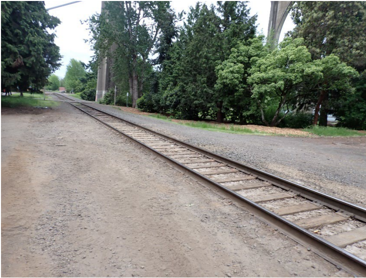
N Bradford Street (railroad ROW) prior to temporary mitigation - view looking southeast. St. Johns Bridge supports visible at the top of photo.
