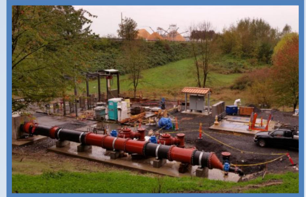
Influent Pump Station
