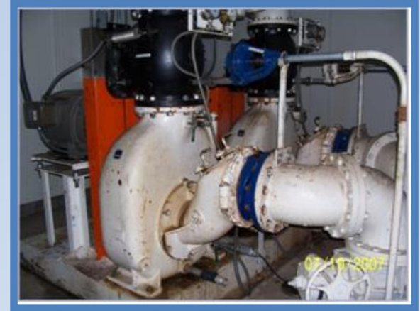
Dayton Station, Existing Pumps
