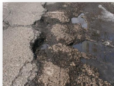
VERY POOR (PCI=20)
