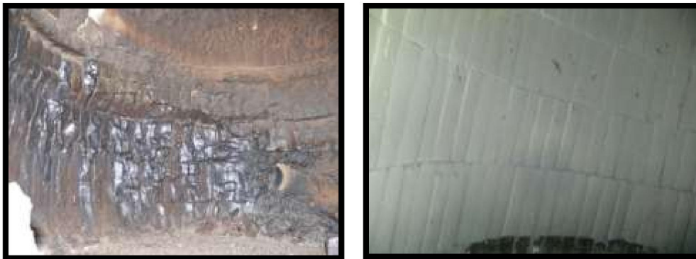
FIGURE 16 DEHYDRATION UNIT BURNER BEFORE AND AFTER CONDITION
