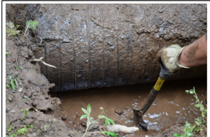
The Dog River pipeline is a 3.5-mile long, 20-inch diameter, wood stave pipeline constructed in the early 1900s using milled pieces of Douglas Fir secured with heavy galvanized wire and sealed with tar.
