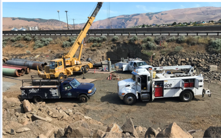
Figure 1: The contractor had to bore under the freeway to install a 36-inch diameter casing in order to install the new 30-inch sanitary sewer main. This picture shows the boring operation on the south side of I-84 in June 2021.
