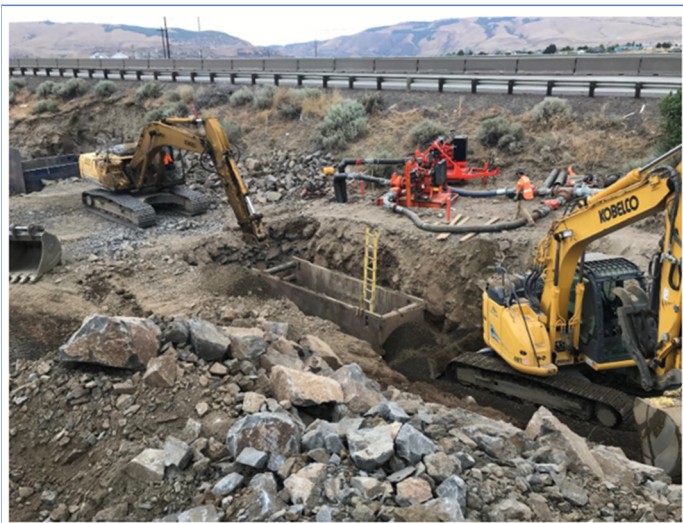
Figure 2: Bypass pumps routed sewer flows to the wastewater treatment plant while the upsized pipe was installed. This picture taken in July 2021 shows the bypass pumps, nearest I-84. A hydraulic hammer breaks up bedrock to the left, while an excavator scoops out a trench on the right. The trench box with ladder in the center keeps workers safe from cave-in.
