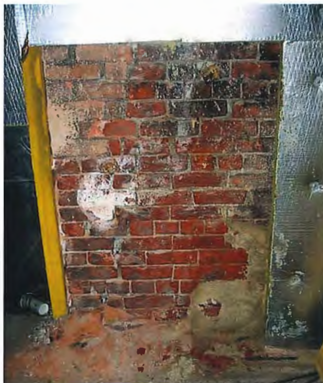
Fig. 21. The interior face of a brick masonry wall shows damage that resulted from the installation of a vapor retardant (foil facing) and thermal insulation. Photo: Simpson Gumpertz & Heger.
