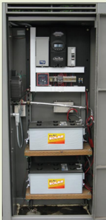
Solar mechanics accessed through rear panel
