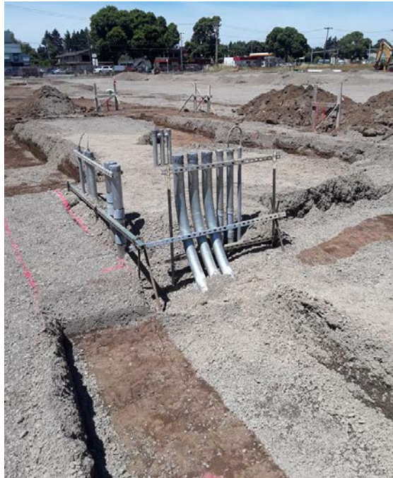
Pictured Above: Batter boards and underground electrical conduit for the driver relief building
