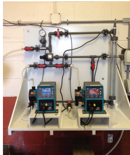
New sodium hypochlorite pumps.
