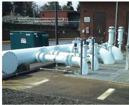
New effluent pumps were put into service in October 2015.
