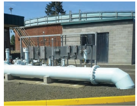
Alternate view of the new effluent pumps.
