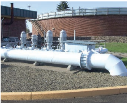
Old above ground turbine pumps and piping.
