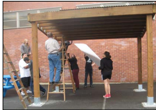
Volunteers Construct Portland Public Schools Bike Shelter. Photo by Anne Laufe with the Oregonian.
