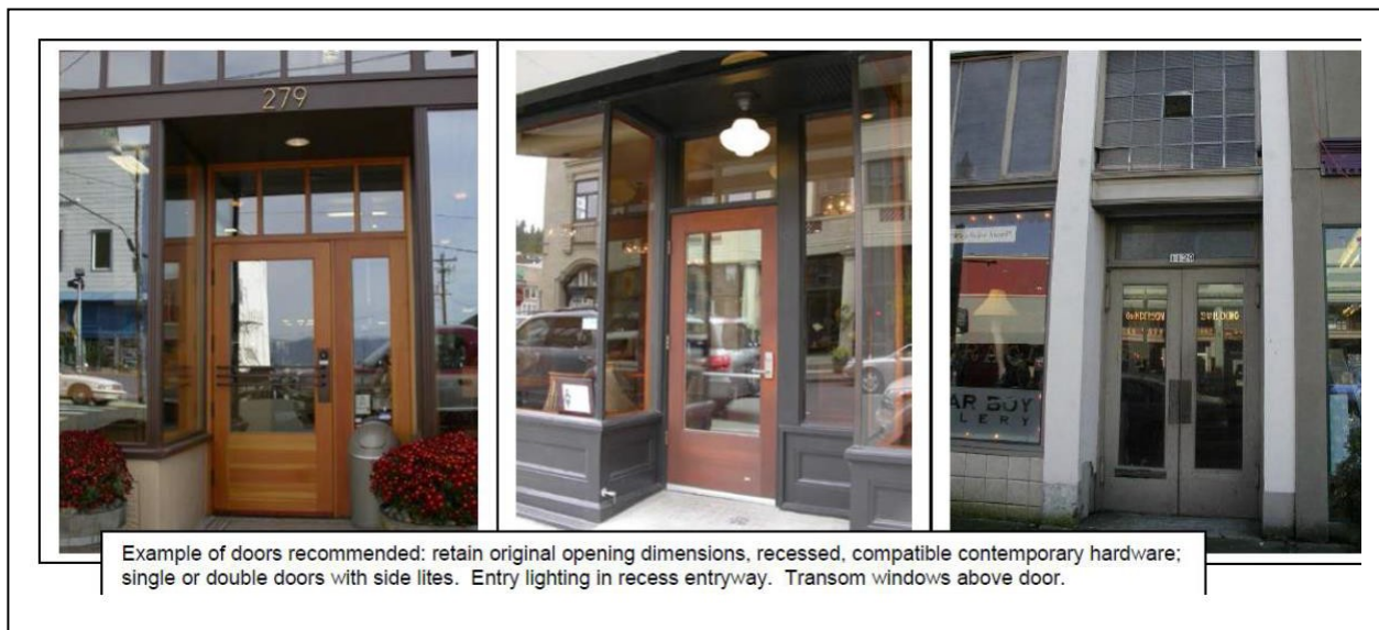
Figure 14.158-11: Recessed Doors, Contemporary Door Hardware, Single/Double Doors, Side Lites, and Transom Windows
