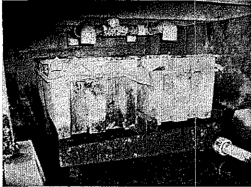
Settling Tanks in Zero Wastewater Discharge system at Mac's in Bend.
