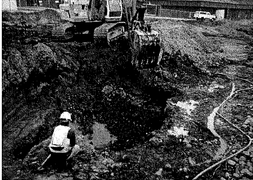
Extra care is taken as contaminated soil is separated and removed from the excavation. (Photo courtesy of Squire Associates)
