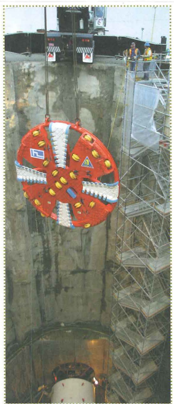
▲ the TBM cutterhead Clark is lowered into the Nicolai Shaft - Clark will tunnel south to connect with the Southwest Parallel Interceptor
