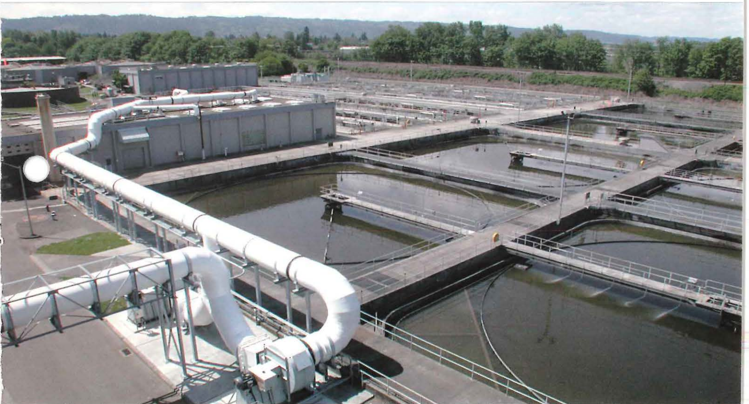
Wastewater Treatment Plant final clarifiers
