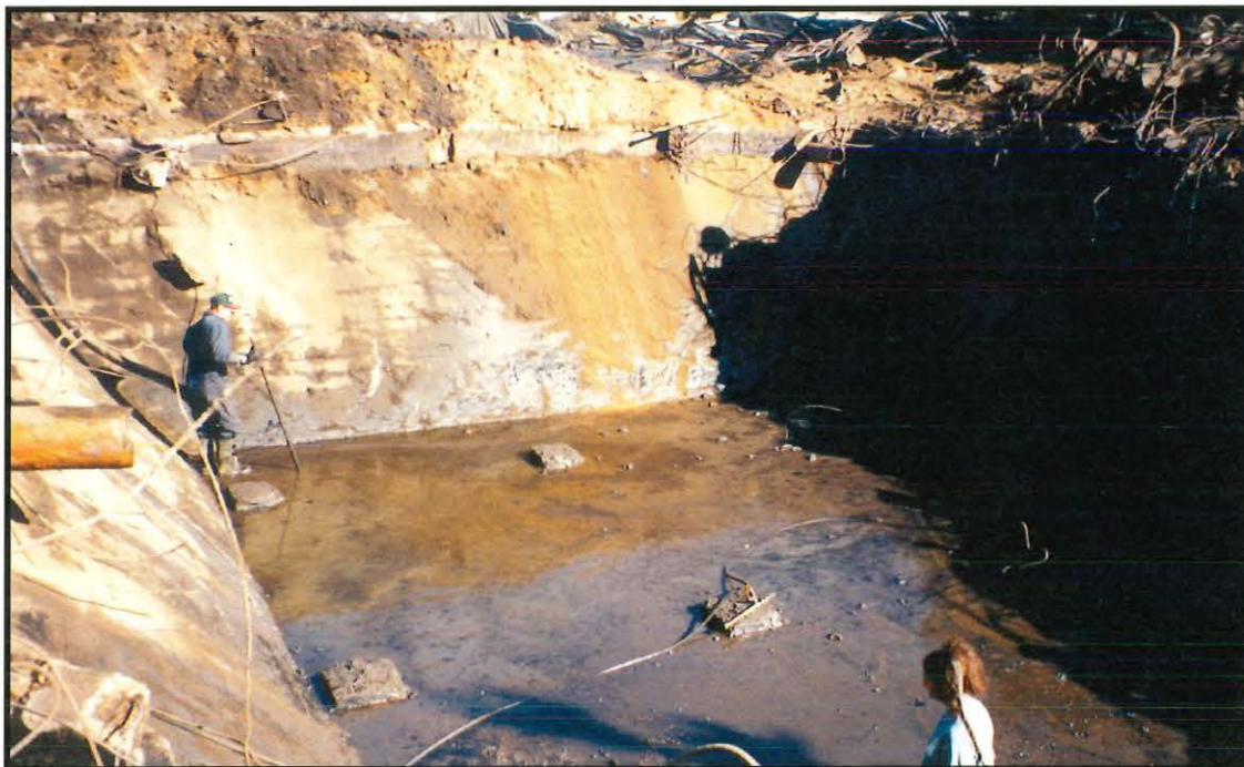
Under the Voluntary Cleanup Program, the facility owner characterized the site and completed initial cleanup activities. The cleanup included removal of an underground storage sump for holding and heating Bunker C fuel.
