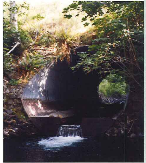
Culvert blocking fish passage on Deep Creek prior to installation of a bridge.
