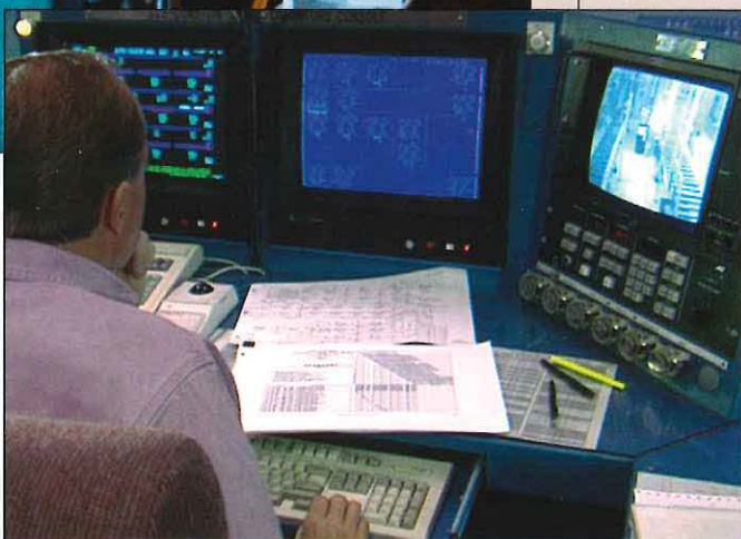
Plant operators monitor and control mechanical disposal processes using control room computers.
