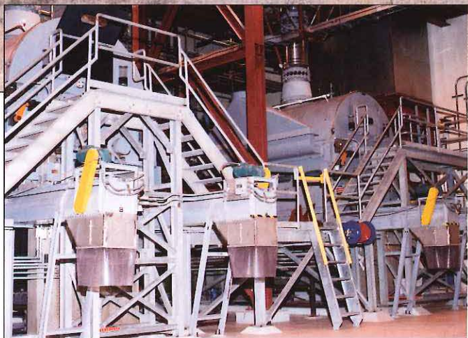
Waste management equipment reduces the volume of liquid waste to a safe and easy-to-handle salt component.
