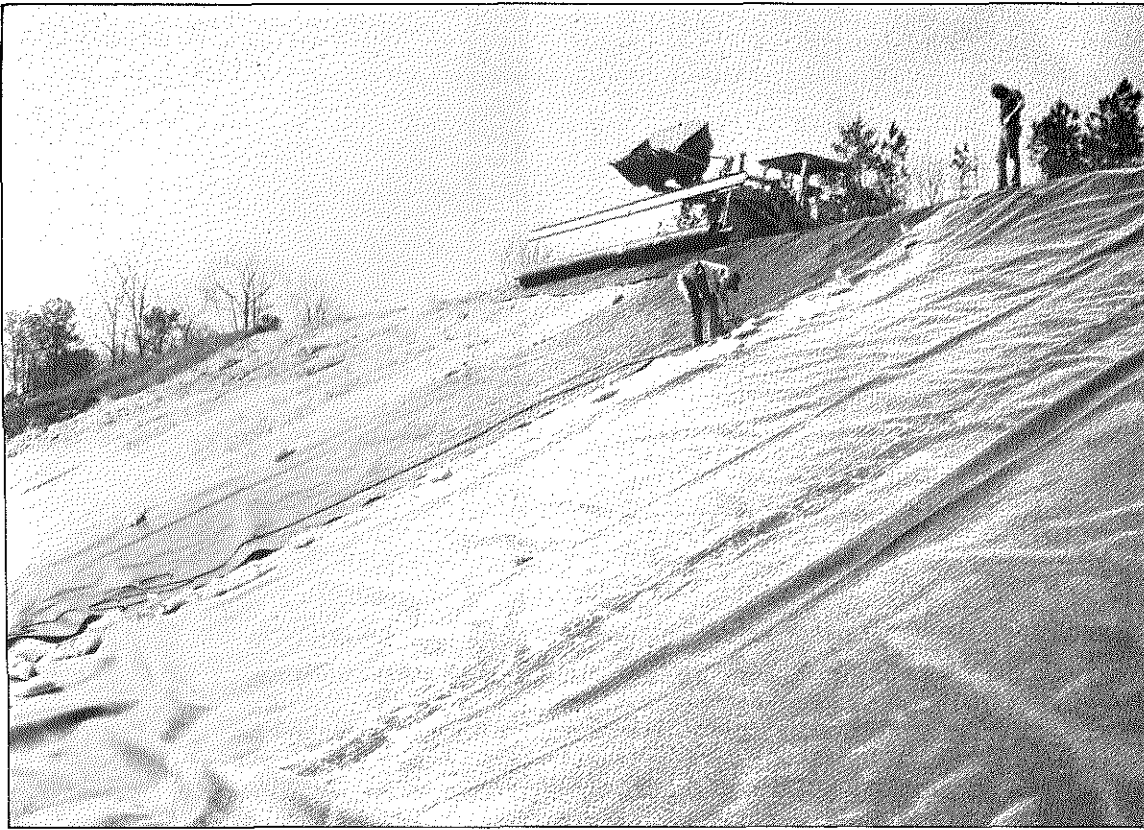
LANDFILL LINER SYSTEM — The bottom of the Gilliam County sanitary landfill will be covered with a high density polyethylene (HDPE) (plastic), similar to the one being installed here at another Waste Management, Inc. facility. The liner is part of the environmental control system designed to protect ground water.
