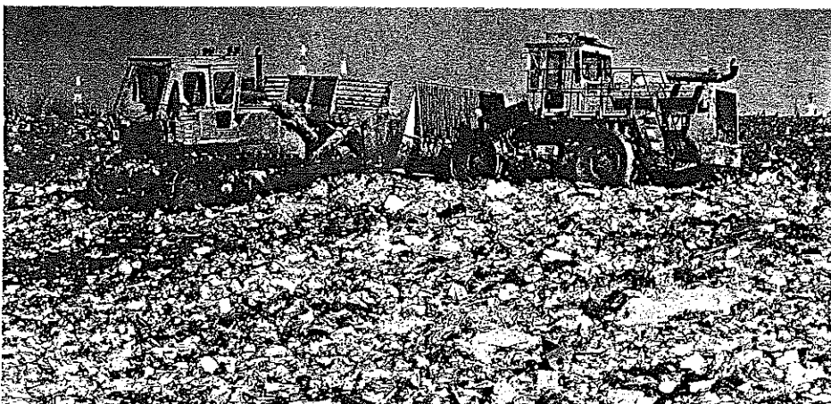
St. John's Landfill could produce enough methane to equal the energy of 63,000 barrels of oil a year.
