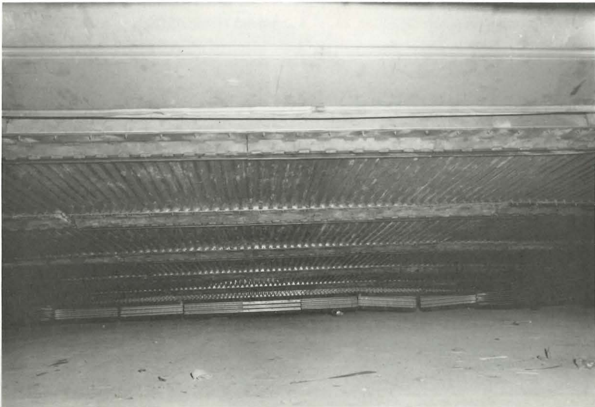
Looking under the cooled-corrugated deck of #75-02 at the multi-air bars typical of #76-05 and #76-06 also.
