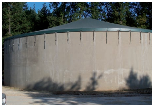
Photo 5: Covered digestate storage tank
