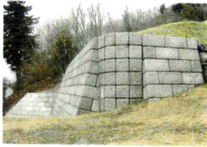
Evergreen Wall Project, Vancouver, WA. Quarry Stone, wedge blocks allow for a wall radius.
