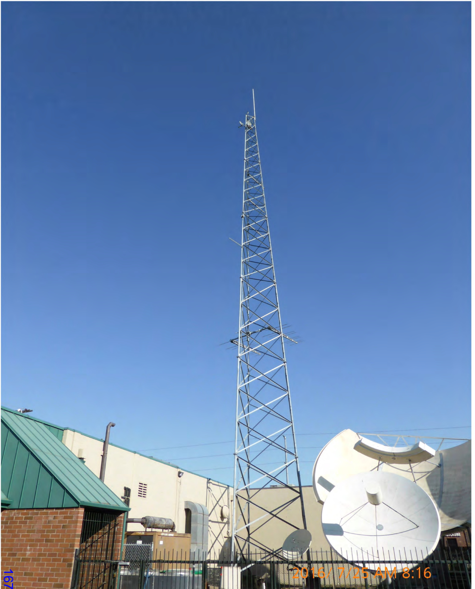
CANBY ID 9, Existing WCF at 144 SE 2nd Ave
