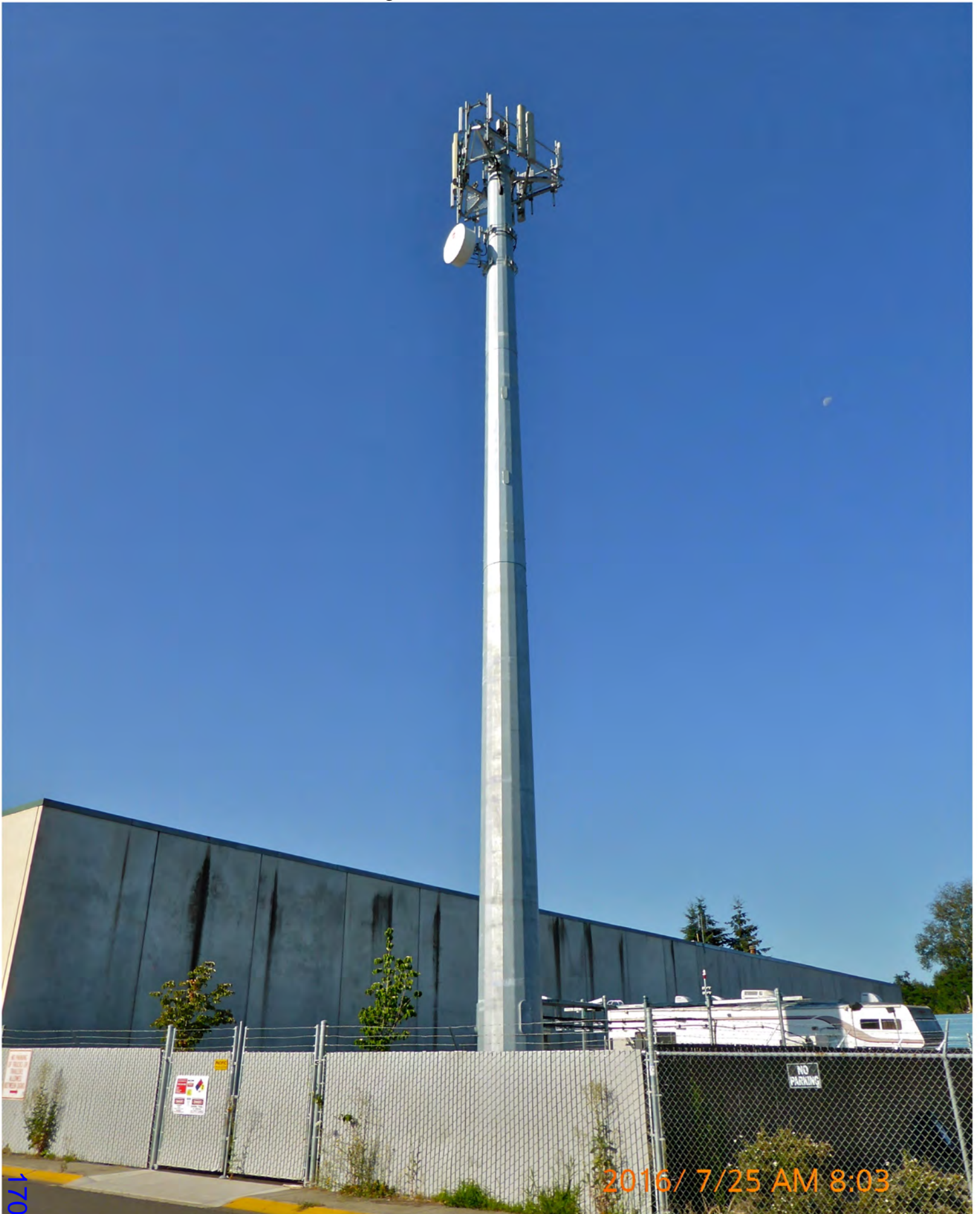
CANBY ID 12, Existing WCF at 1190 NW 3rd Ave, faces Baker Rd
