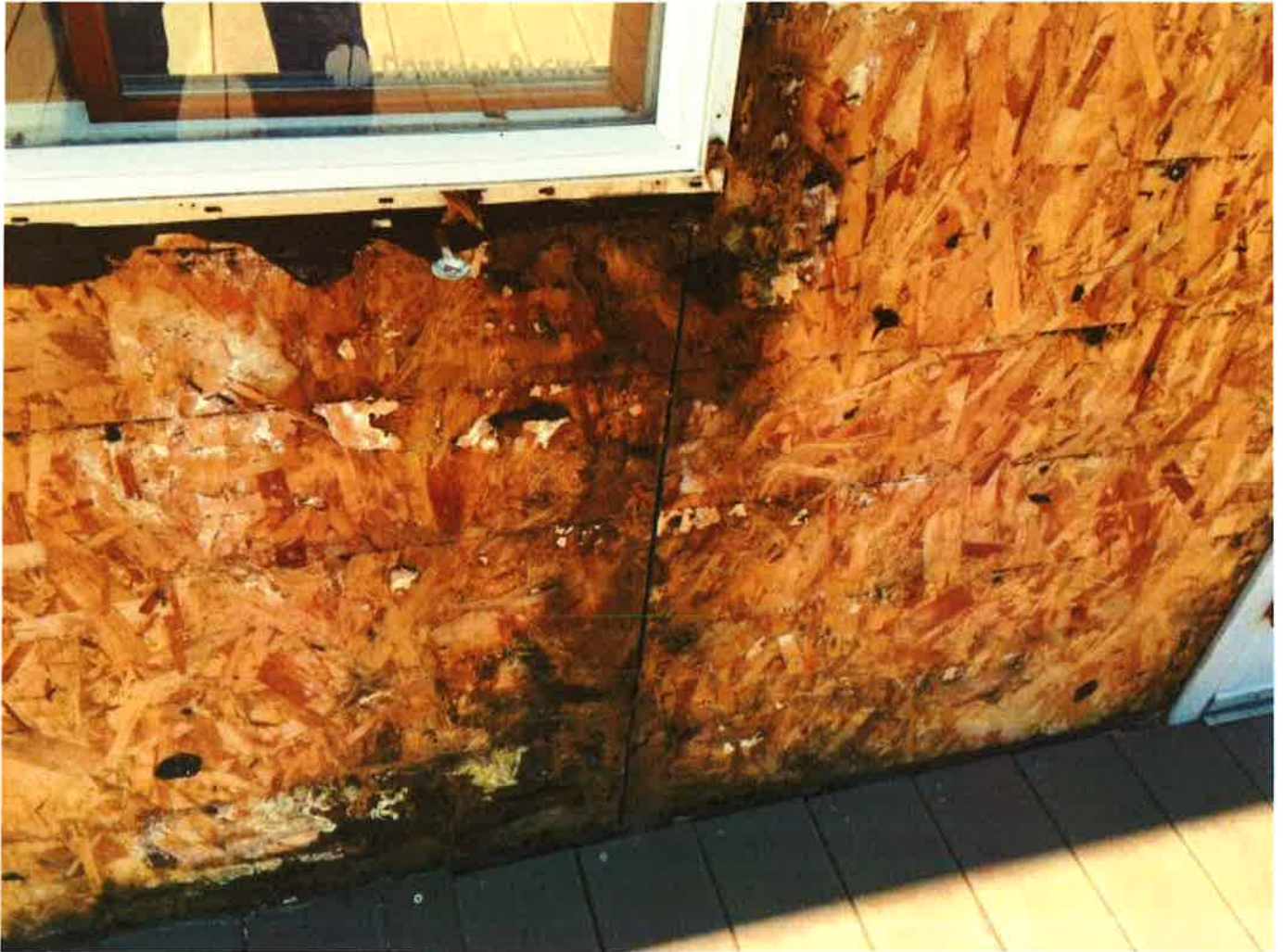
17 29-IMG_0518 Date Taken: 6/6/2016 dry rot under window extending below deck.
