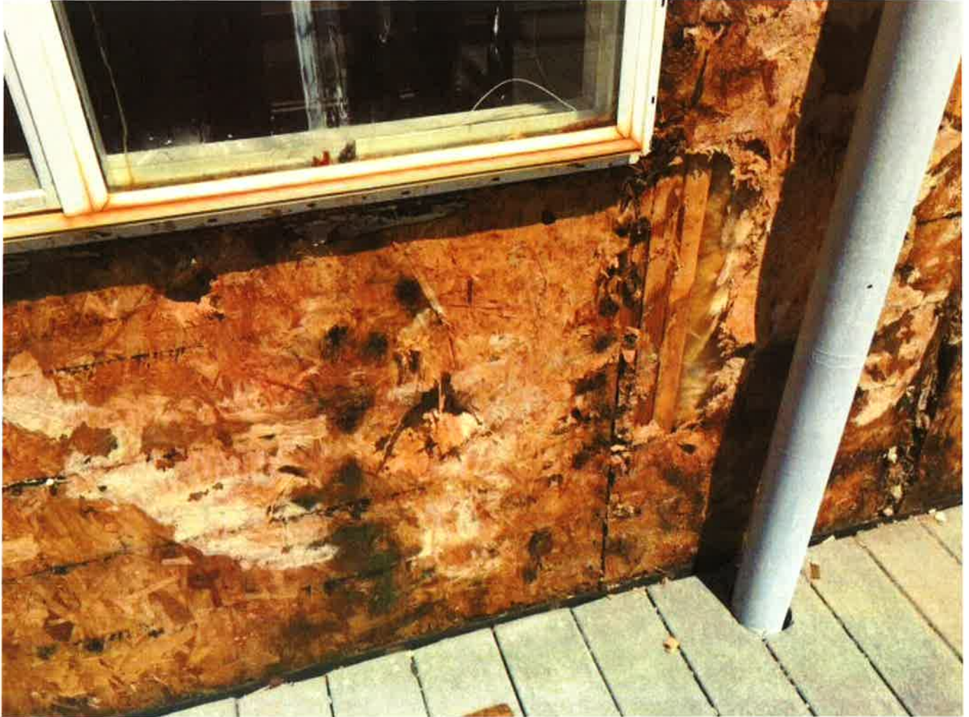
8 20-IMG_0509 Date Taken: 6/6/2016 mildew and dry rot under a window and along deck extending under deck
