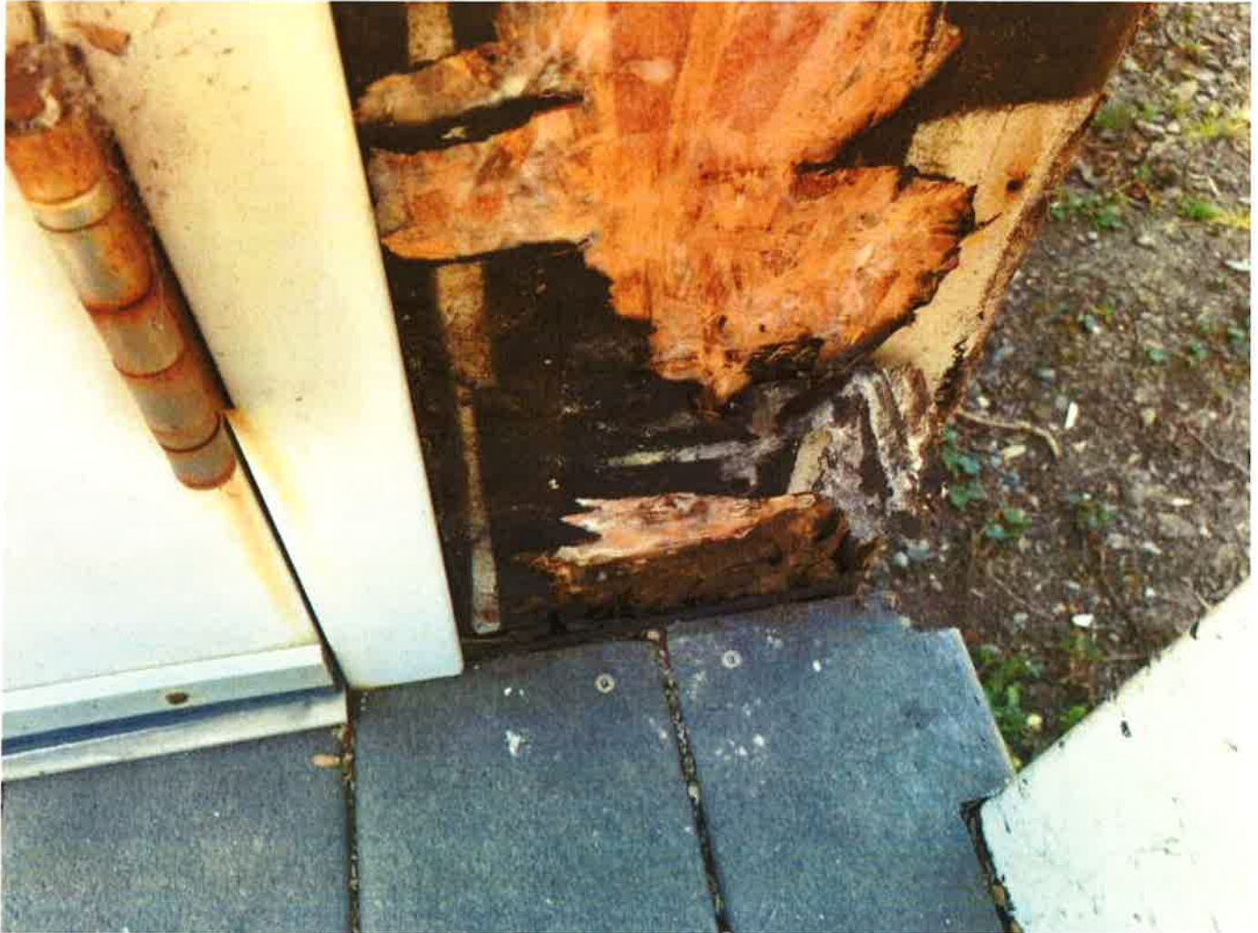
29 41-IMG_0530 Date Taken: 6/6/2016 Water damage on corner of building.
