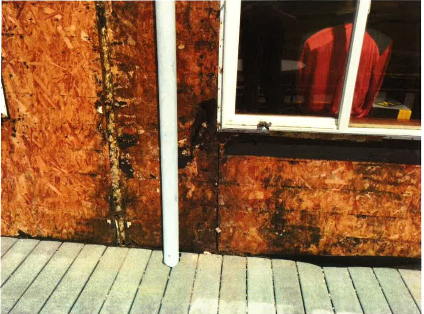
13 25-IMG_0514 Date Taken: 6/6/2016 dry rot around window extending below deck
